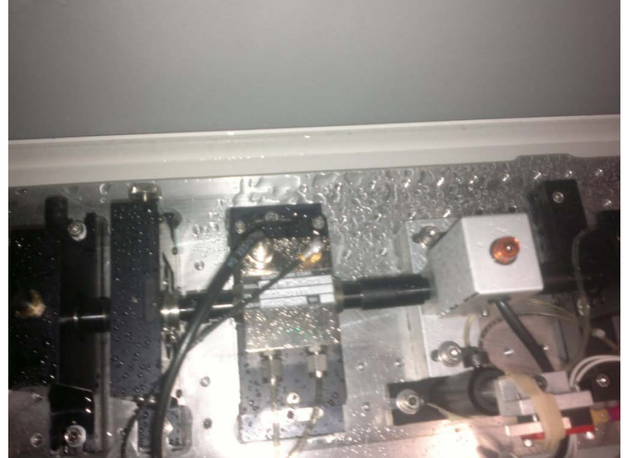
Broken flow tube → Water leak
